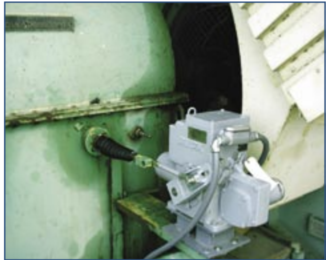
Raw Mill Dust Collector Fan Speed Control
