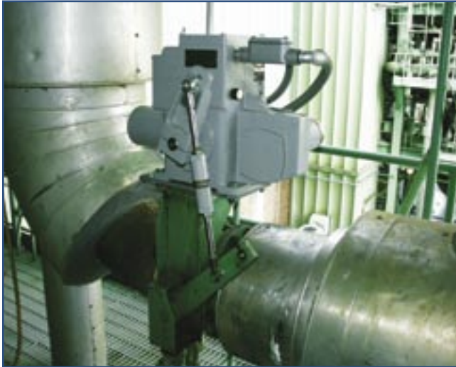
Main Fuel Gas Valve
