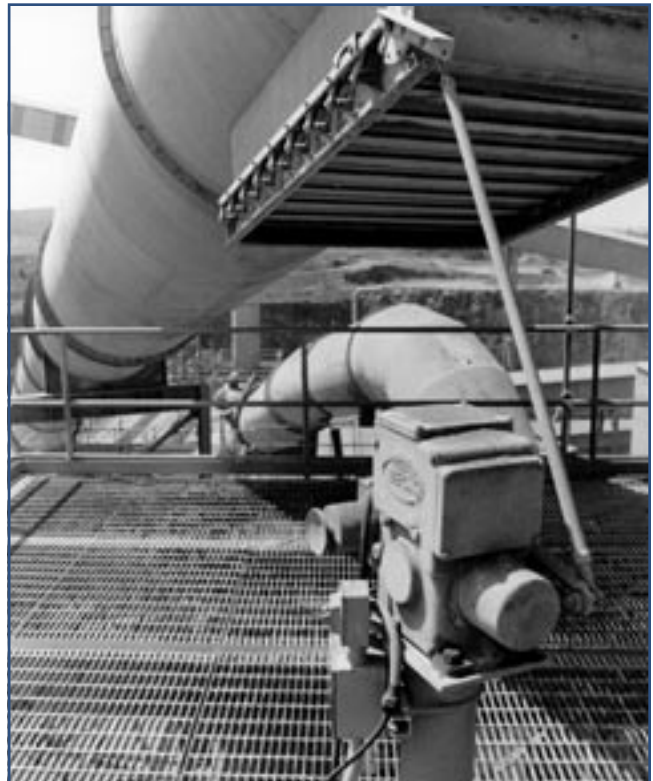
Baghouse Tempering Air Damper
