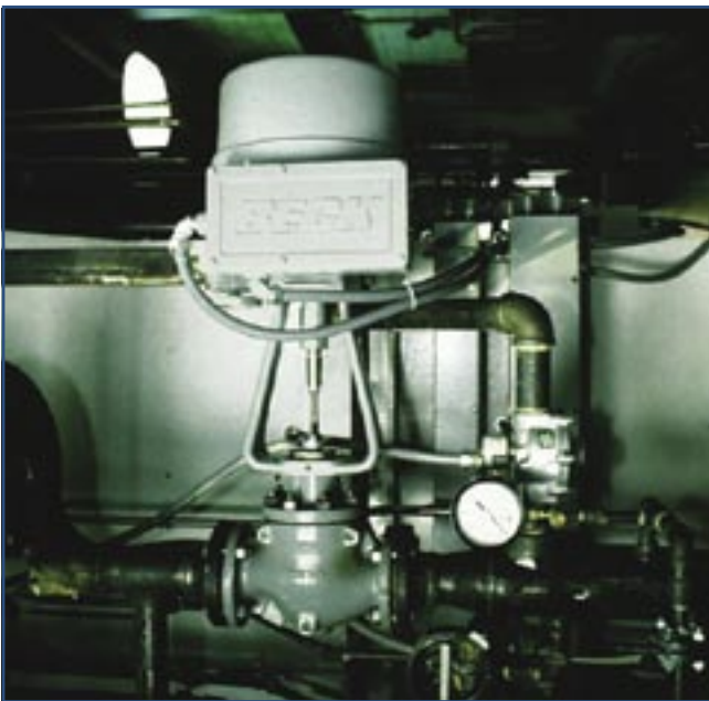
Kiln Fuel Oil Valve
