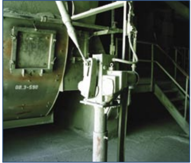
Primary Air Fan Damper
