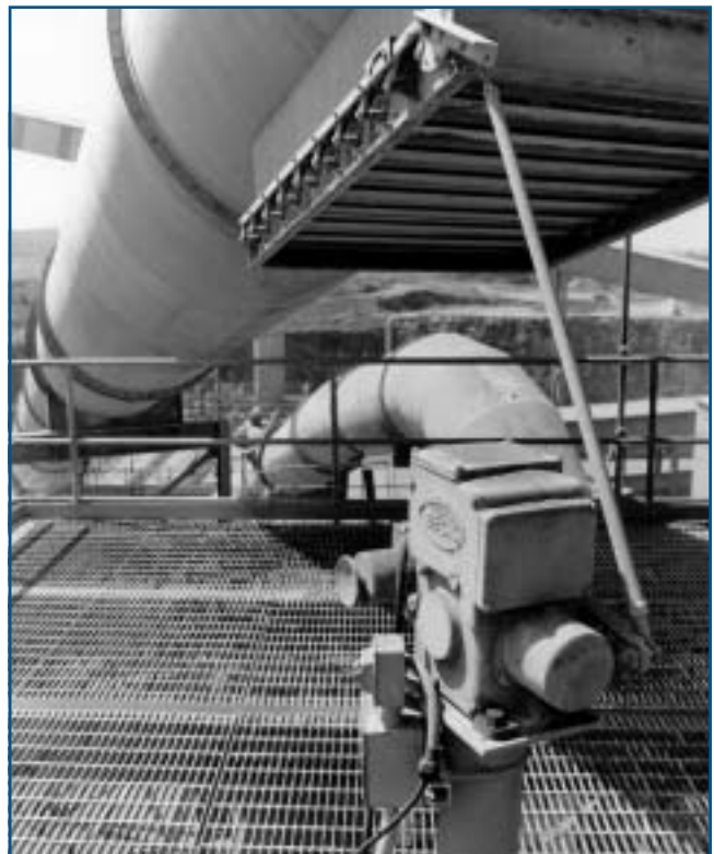
Baghouse Tempering Air Damper
