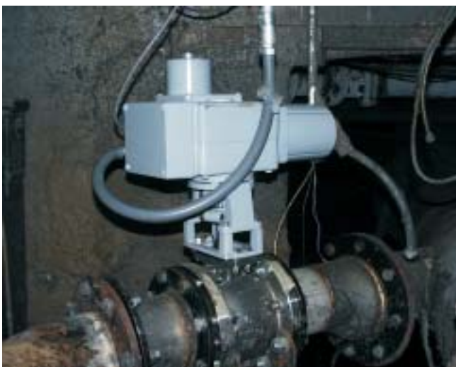
Vat level control valve
