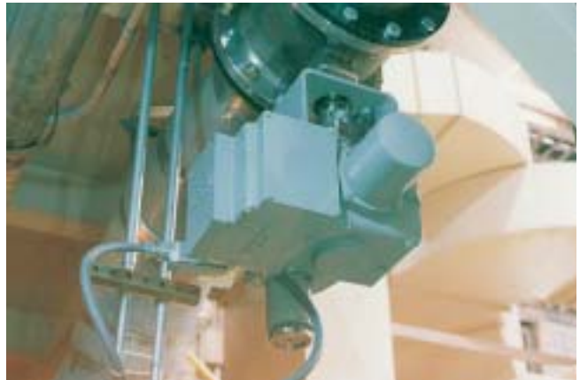
Stuffbox level control valve
