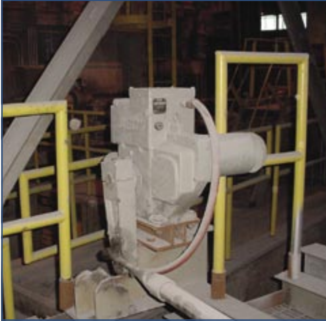
Reheat Furnace Exhaust Damper
