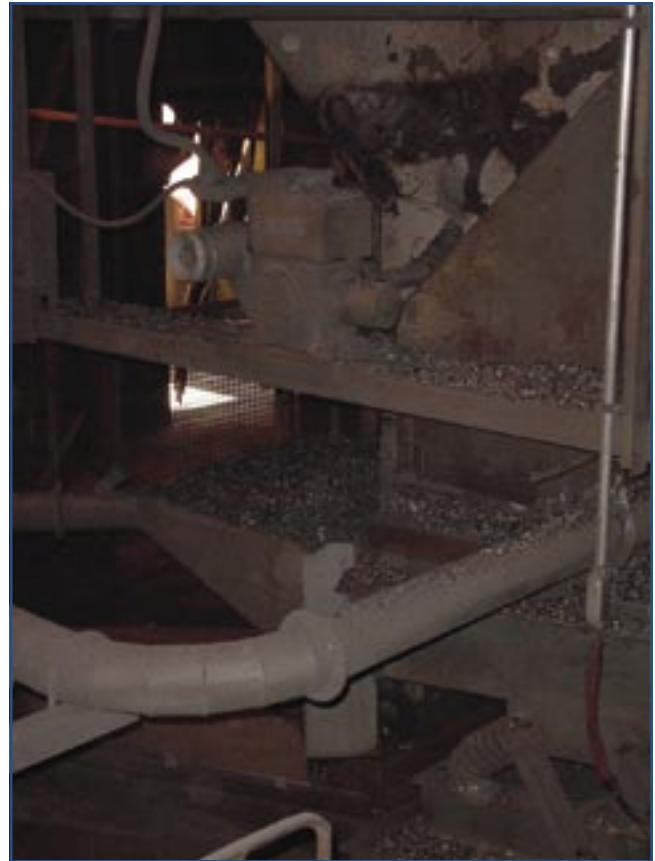
Sinter Plant Fines Gate Control
