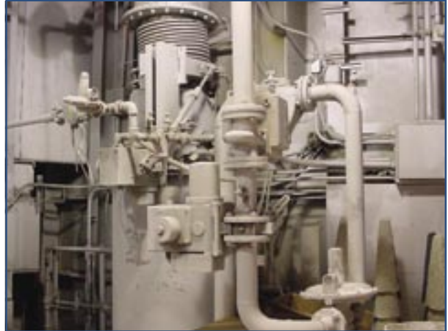
A & P Line Gas Valve
