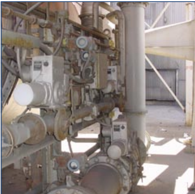
Stove Enrichment Gas Valves
