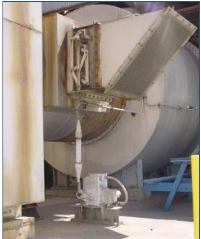
Melt Shop Fume Control Tempering Air Damper
