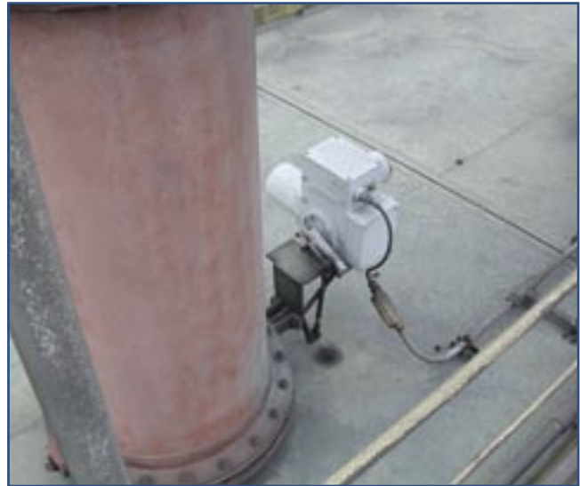
Lime Kiln Primary Air Damper
