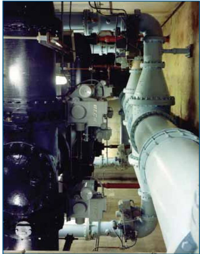
Multiple Beck drives on flow control valves
