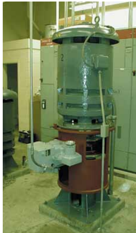
Beck Model 11-200/300 installed on a MagnaDrive Vertical ASD
