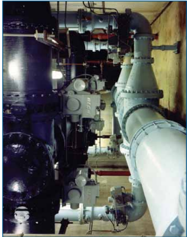
Multiple Beck drives on flow control valves
