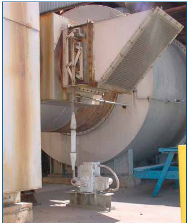
Mixing Air Bottom Damper
