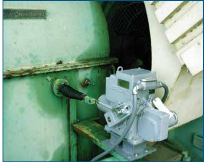
Raw Mill Dust Collector Fan Speed Control
